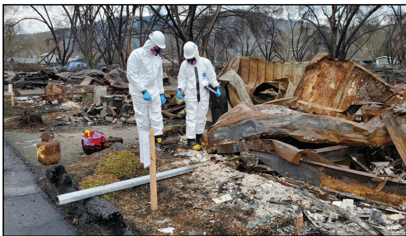
Crews gather samples to test for asbestos in the Alameda Fire area
