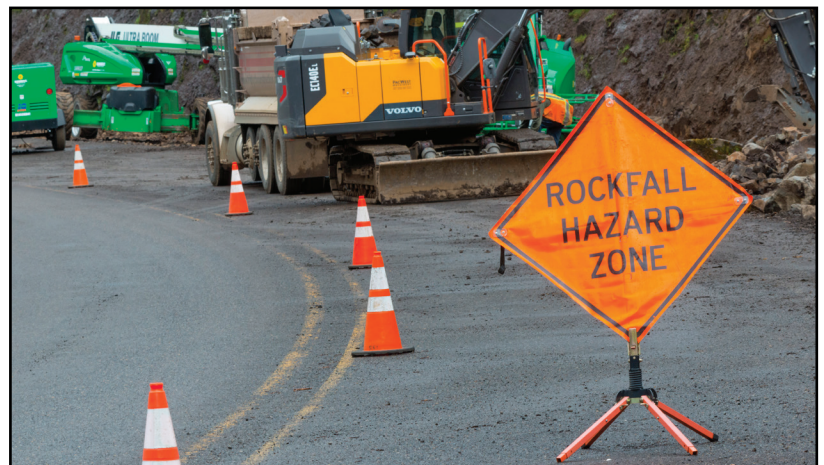
Rockfall hazard zone along OR 224
